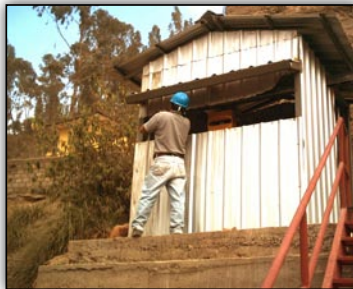
The Centurion Installation at Guapan
