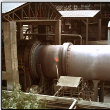
Hotspot clearly visible on the Kiln Shell
